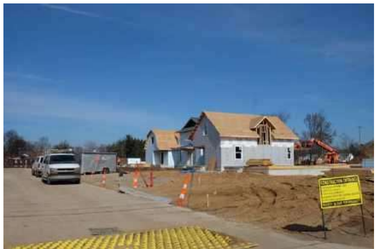
Affordable housing units under construction at the Community Land Trust located at 2080 Union Avenue.
