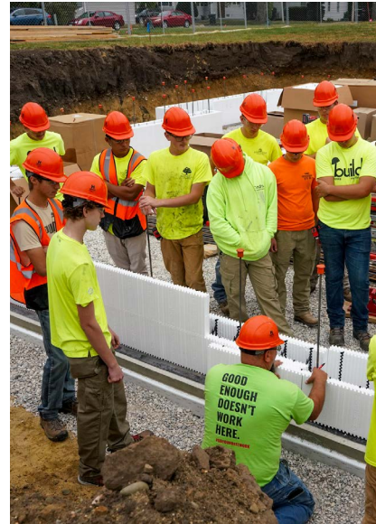
First-year students in the Sustainable Construction and Design program at Hawkeye Community College in Waterloo, Iowa, learn about building a foundation. Photo courtesy of Hawkeye Community College.
